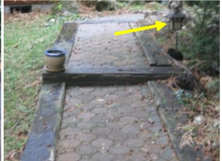
Interlocking brick walkways and exposed aggregate sidewalks are the surface area of all exterior walk ways. They are in good condition with lighting at all steps.
