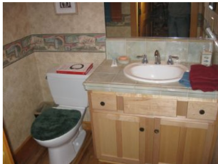
Bath #3 maple cabinet and hardwood floor.China lavy and toilet all functioning properly when inspection was made.
