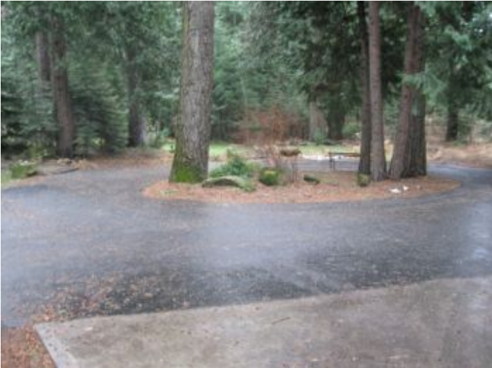
Asphalt driveway in good condition. Concrete apron poured in front of all garage openings with proper slope for water.
